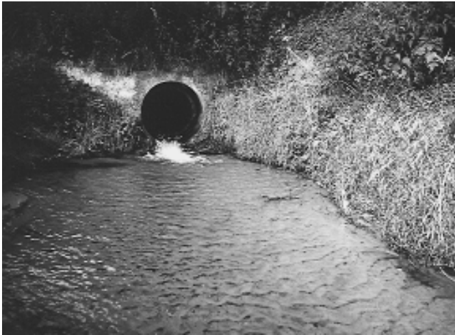
Figure 4.14. Falls evened out at culvert outlet. In cases where the outlet of a culvert, e.g. at a road underpass, is higher than the stream water level (left), one can establish a short riffle or lower the culvert to the level of the stream (right).
